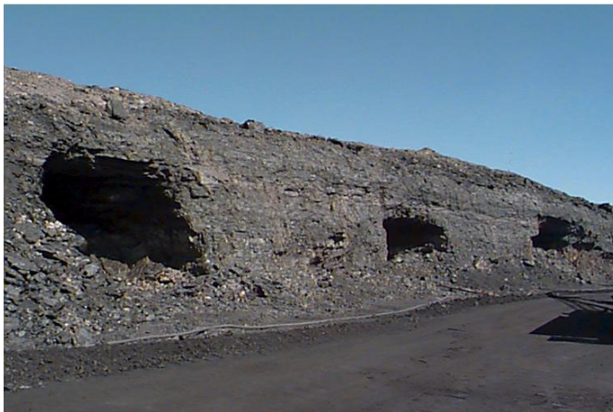
Figure 11: Open bords when buffer blasting is not practiced or the buffer has been excavated
